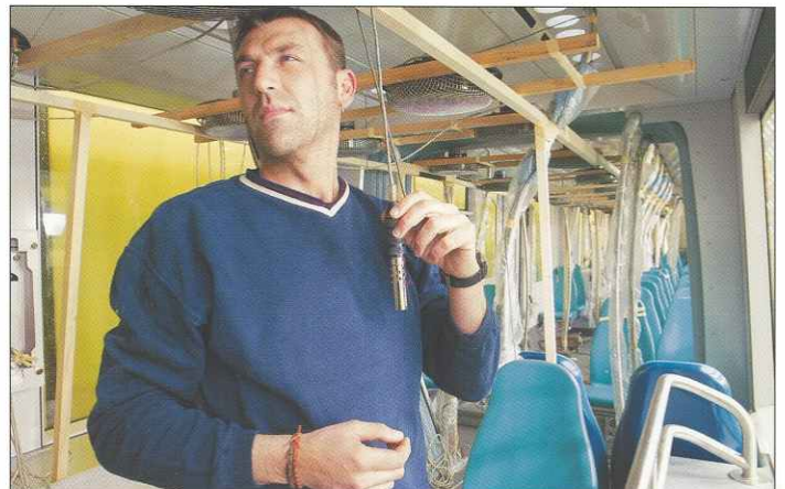
Installation of temperature sensors in CITADIS preparing the final k-value measurement. The k-value is a heat transfer coefficient, describing the heat transfer of the air from the interior through the walls to outside.
